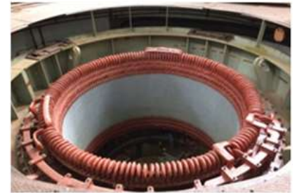
NEWLY REWOUND 30MW HYDRO GENERATOR AT UMIAM STG-III HYDRO PROJECT
