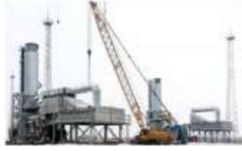
35 MW GT POWER PLANT, KAZAKSTHAN
