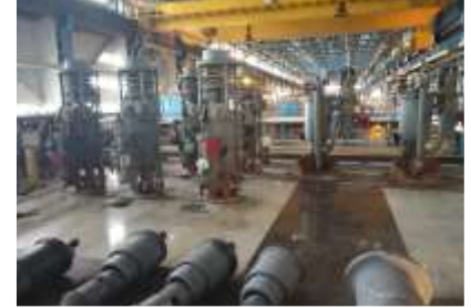
CONTROL & STOP VALVES OVERHAULING SIPAT 660MW
