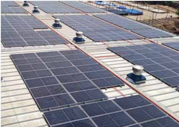
Solar Plant at Cuttack
