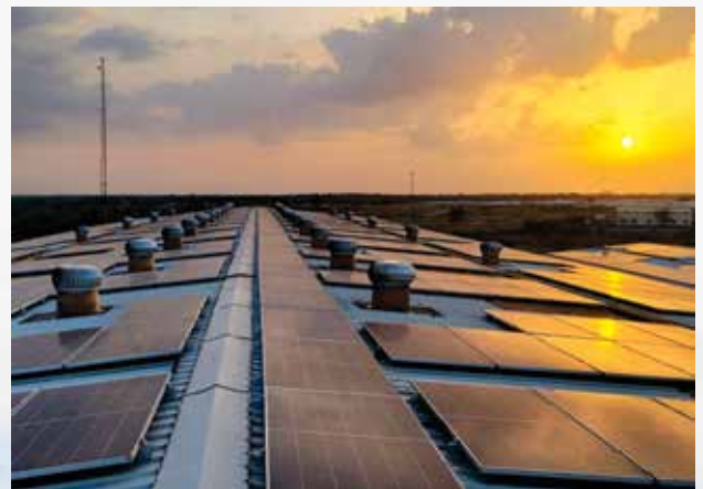
Solar Plant at Halol Composite
