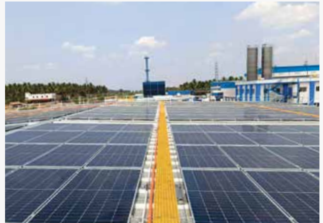
Solar Plant at Erode
