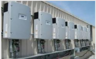
String Inverter Huawei /Sungrow Total of 460 MW
