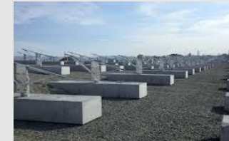
Ballast Foundation Total of 51 MW
