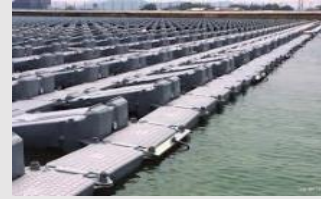
C&T Total of 427 MW
