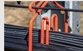
CAB System Total of 28 MW
