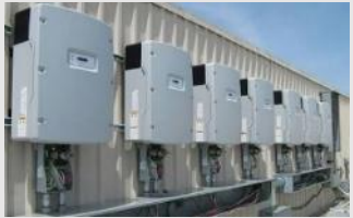
String Inverter Huawei /Sungrow Total of 460 MW
