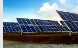
2P Soltec, Arctech, ATI Total of 390 MW
