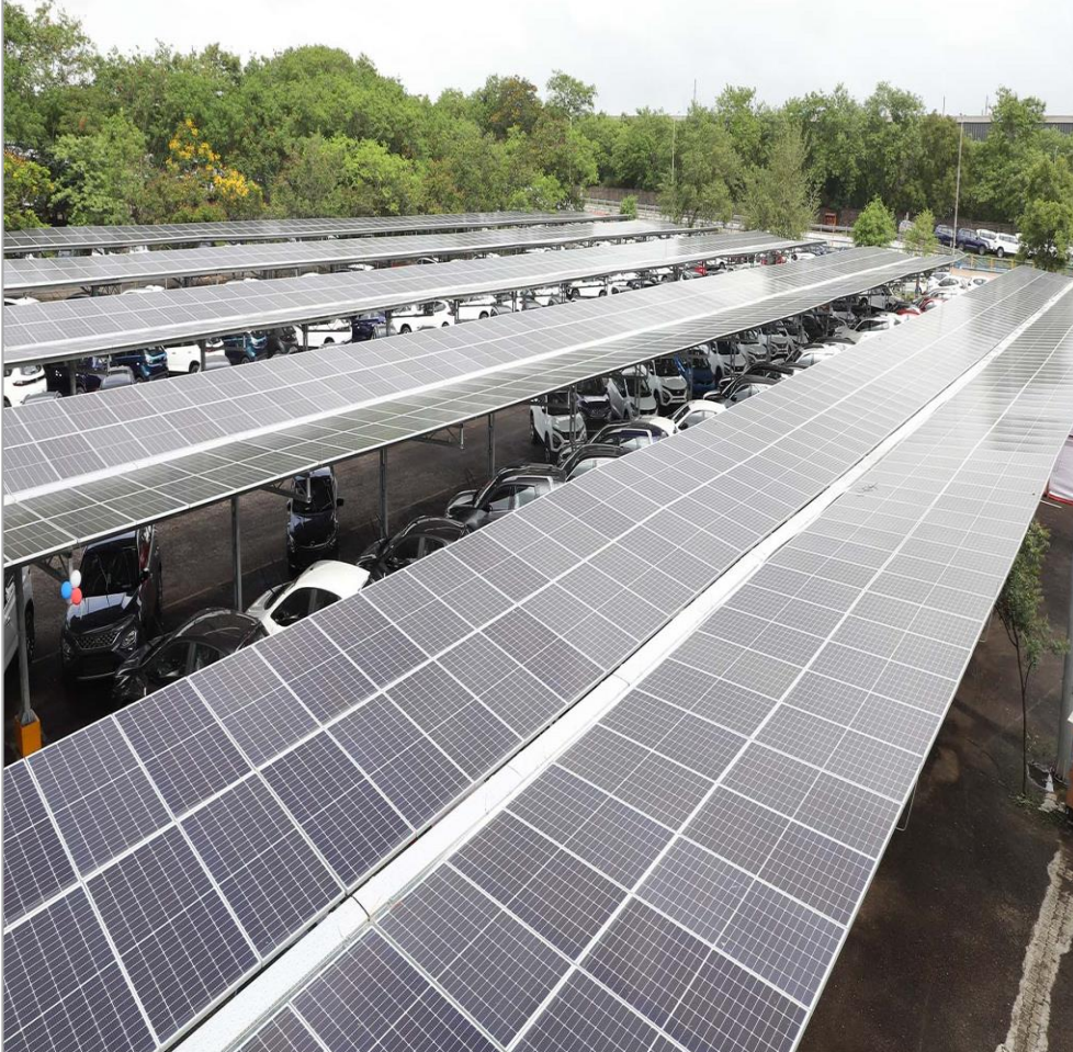
6 MW Carport Installation at Tata Motors, Pune India's largest grid-synchronised, solar carport
