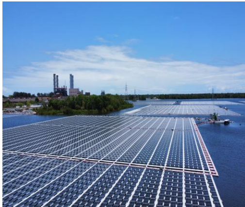
70MW NTPC Kayamkulam, Kerala - One of the largest floating solar in the Country
