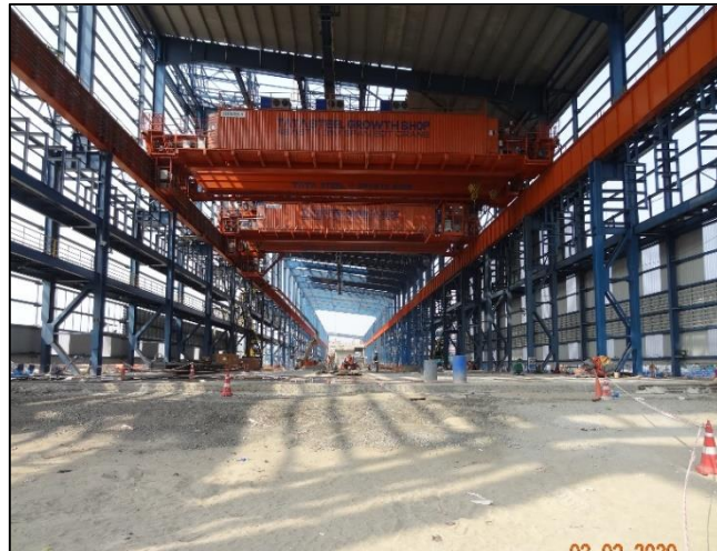
EOT Crane of PLTCM
