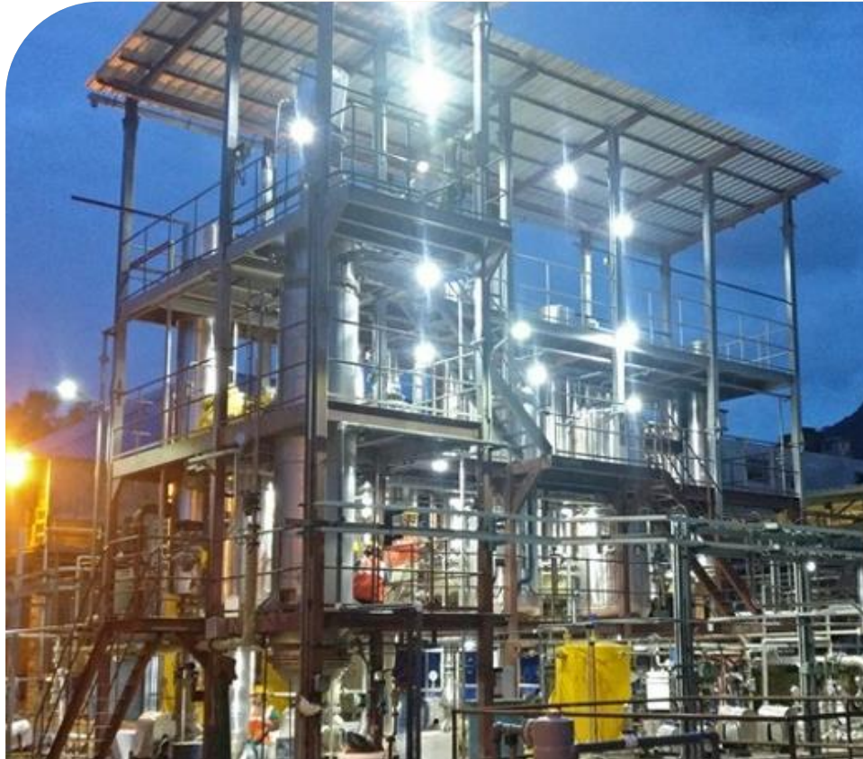
3.75 MLD Zero Liquid Discharge plant for a textile major
