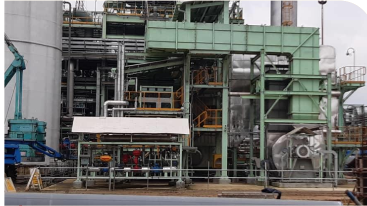
Remote commissioning of 125 TPH FM boiler at Indorama, Nigeria
