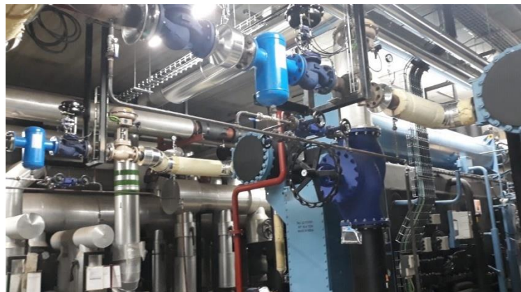
Remote commissioning of two double-effect steam fired chillers of 3MW cooling capacity in Spain
