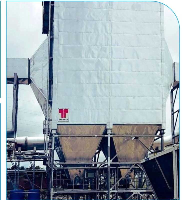
Remote commissioning of an ESP on a husk fired boiler in the Philippines
