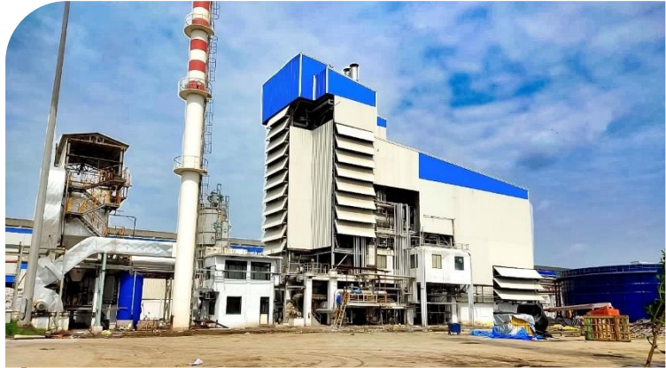
First-of-a-kind non-recyclable solid waste fired boiler at a paper mill
