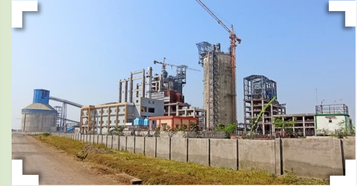
1.8 mtpa greenfield grinding unit at Dhule, Maharashtra, taking cement capacity of the Company in the state to 19.45 mtpa.
