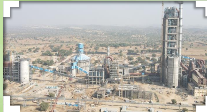
1.9 mtpa integrated cement unit at Pali, Rajasthan, taking cement capacity of the Company in the state to 16.25 mtpa.
