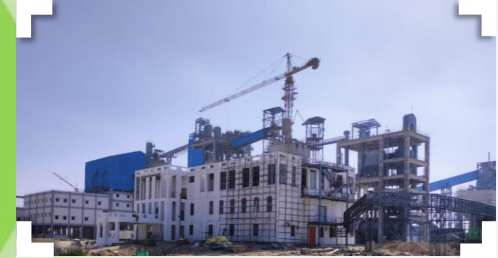
0.4 mtpa greenfield wall care putty plant at Nathdwara, Rajasthan. UltraTech now has a wall care putty capacity of 1.3 mtpa in India.
