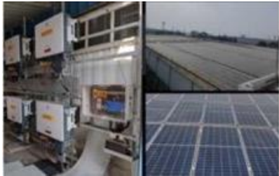
4W Switch Plant Pune
