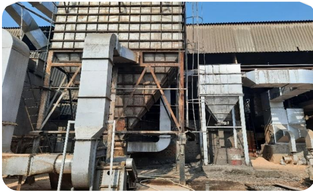
Thermic Fluid Heater
