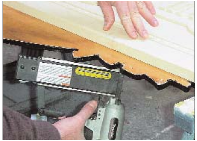
Using a brad nail gun, we nail the perimeter of the sign to hold the HDU in place while the epoxy cures.
