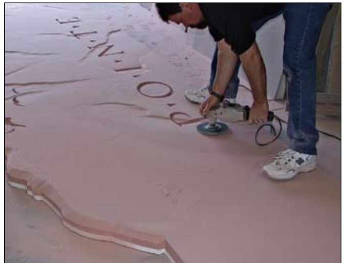
Here I am bending over the slab with the L-head grinder. Fortunately for my back this step was complete in about 1 1/2 hours.
