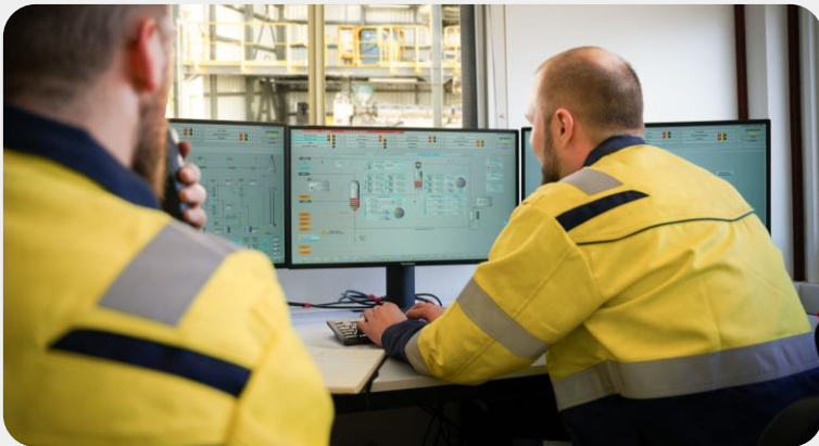
Actual control panel of the Demo Plant, monitoring over 300 parameters to ensure process stability and operational safety
