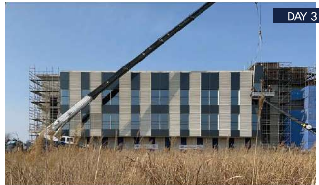
New Construction of National Energy Technology Laboratory Total Operation Center (March 2025, Saemangeum, South Korea)
