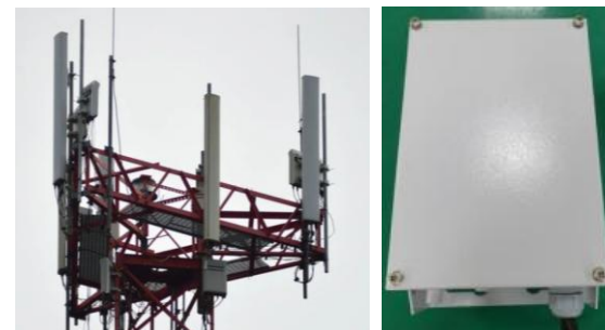
Telecom | Overseas & Domestic
