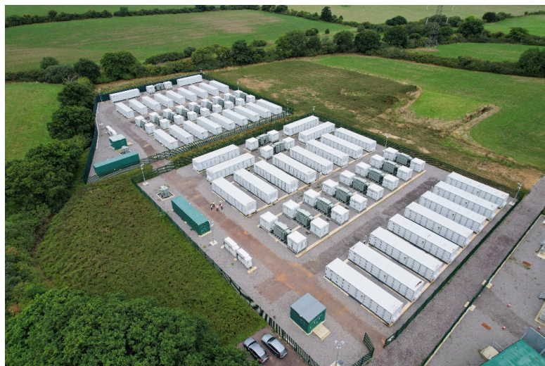
Minety Battery Storage Station in UK (100MW/100MWh), 2021
