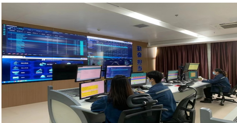
China's First PV Monitoring System
