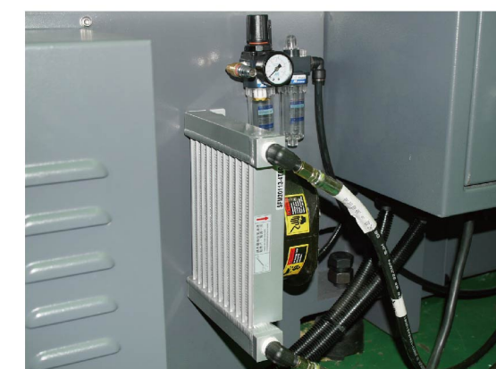
The cooling system for Hydraulic system
