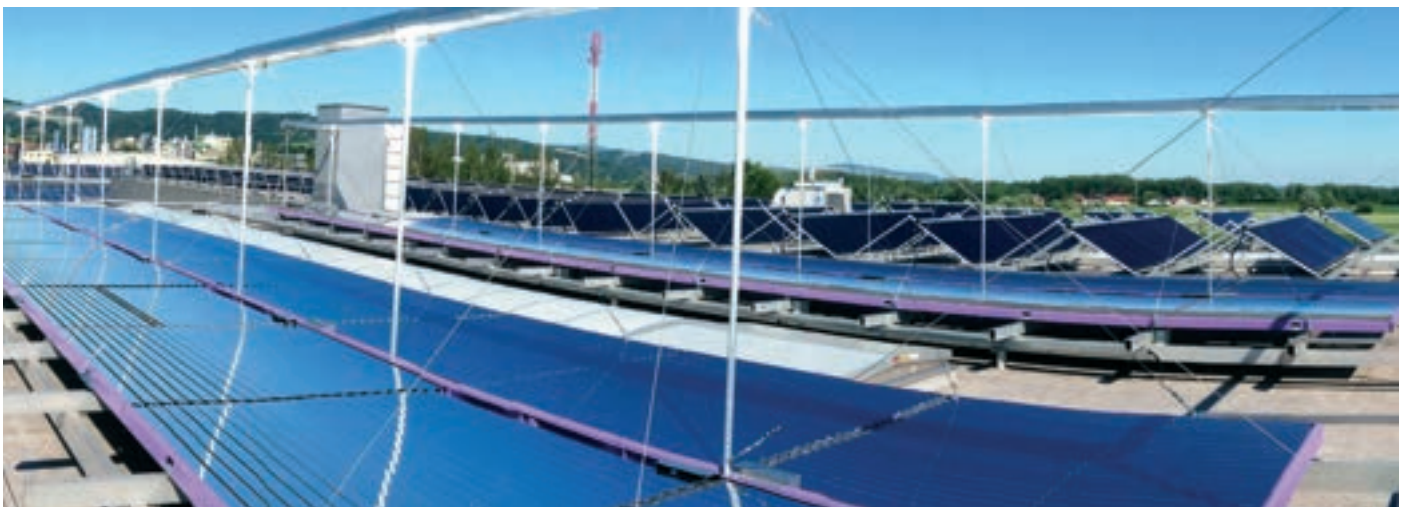
400m² ECOTHERM Fresnel / Flat Plate / Solar Field for heating and cooling at the roof of our ECOTHERM headquarter
