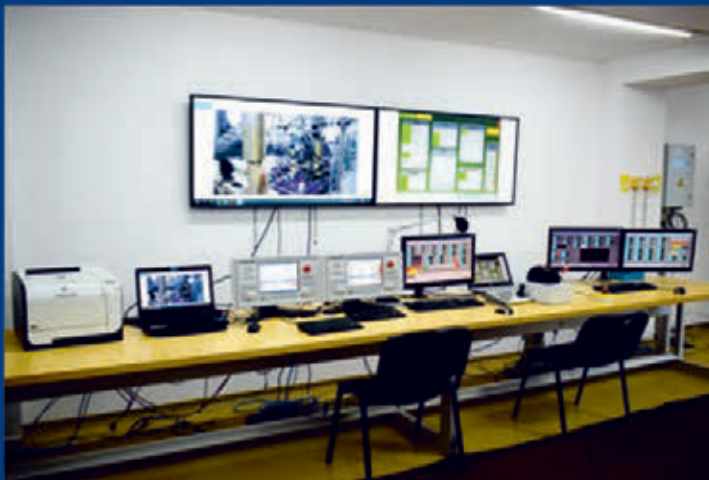
Test banch control room.
