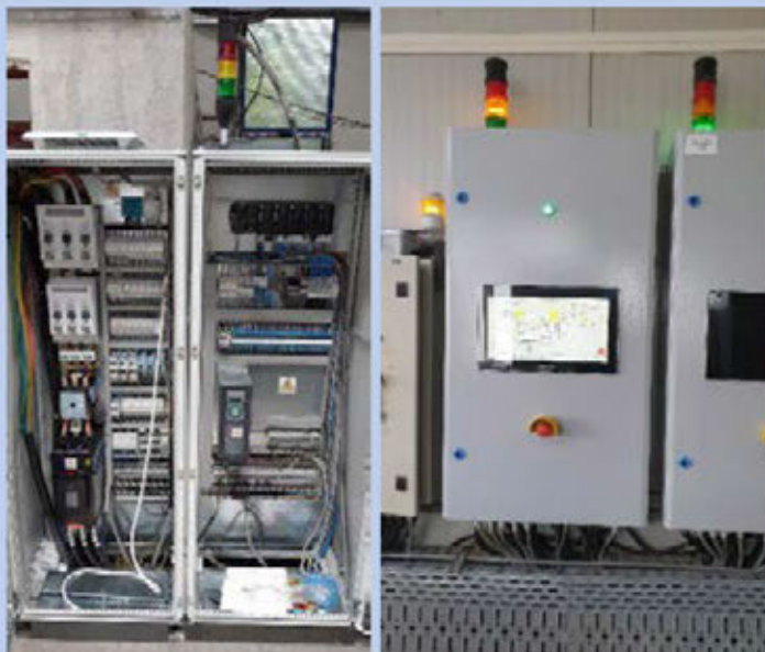
Automation cabinets for compressors, installed in control rooms within stations for oil and gas industry
