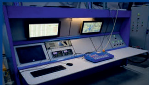
Auxiliary control and instrumentation unit.
