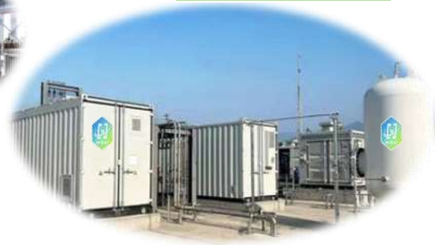
Manufacture factory and Operation site
