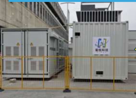
MW level System testing
