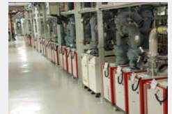
Pumps, vacuum pumps
