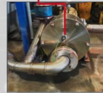
Sensors placement on pump and filter for pumping processed old paint
