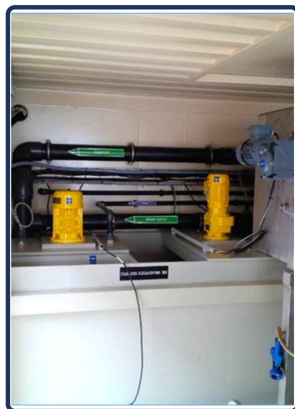
Cuves coagulation / floculation
