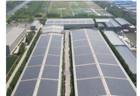
200MW Distributed PV Project in Hebei
