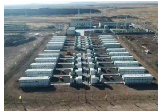
60MW/120MWh BESS Project in Neimenggu
