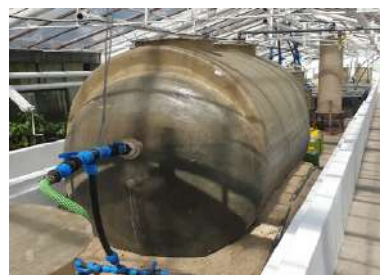
5 m 3 digester – Complex project 32PCCDI/2018
