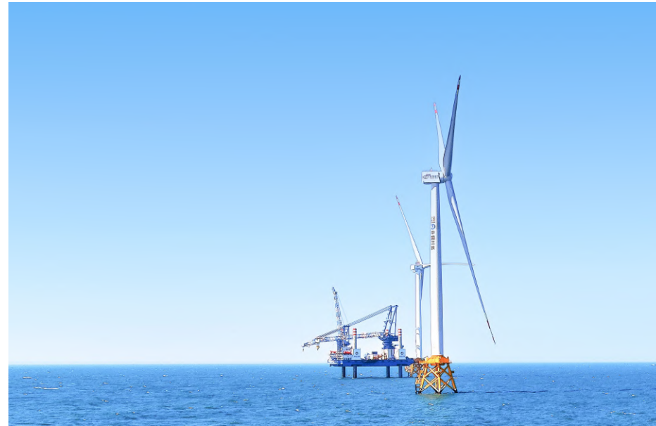
Offshore Wind Farm in Fujian, ZhangZhou 13MW Wind Converter Batch Application
