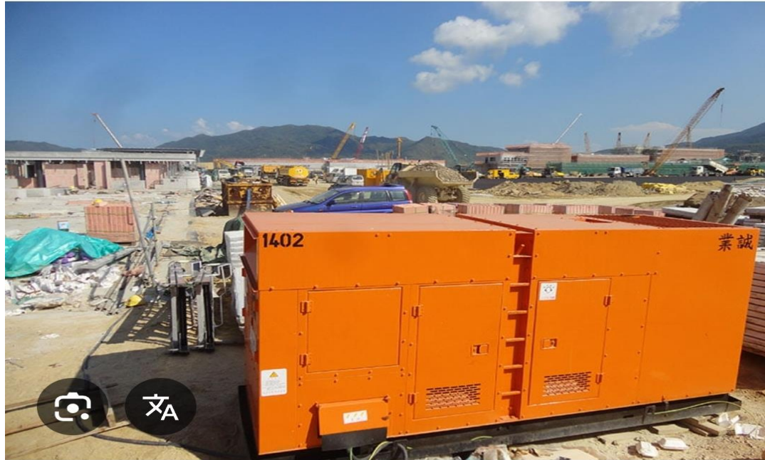
Diesel Generators Hong Kong - Yip Shing Diesel Engineering Co.,...
