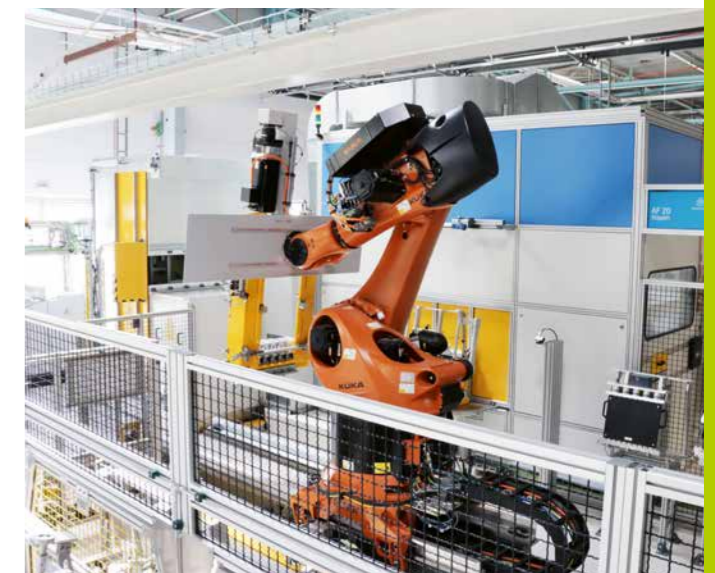
Automated stacking machine for the production of PEM electrolysis stacks at the Wasserstoff Campus Salzgitter.
