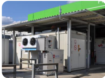
High pressure test bench
