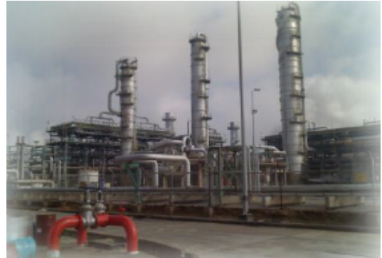
Gaz Oil Stations
