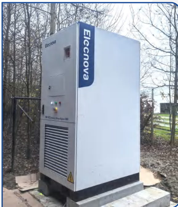
Date: 2024.06 Model: ECO-E233LS Project Volume: 100kW/233kWh
