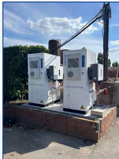
Date: 2025.08 Model: ECO-E107WS Project Volume: 100kW/214kWh
