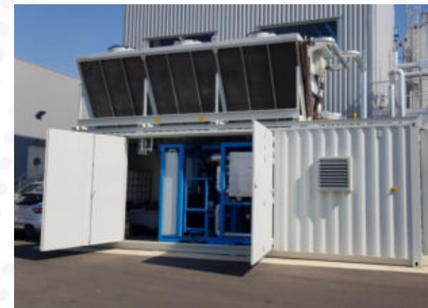
Heat recovery on Incinerator– 180kW ORC - France
