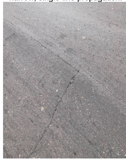
Figure 4 — Crack intersecting a construction/transverse joint line.
