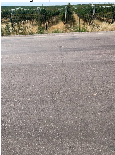
Figure 3 — Crack extending toward the shoulder edge; no adjacent alligator cracking observed.
