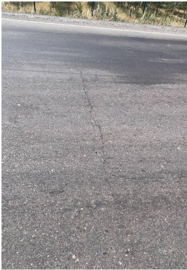
Figure 1 — General view of the longitudinal crack along the pavement lane.
