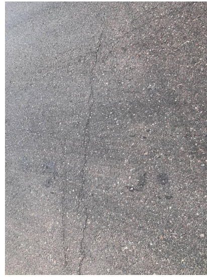
Figure 2 — Close-up of the crack line showing narrow, single-line propagation.
