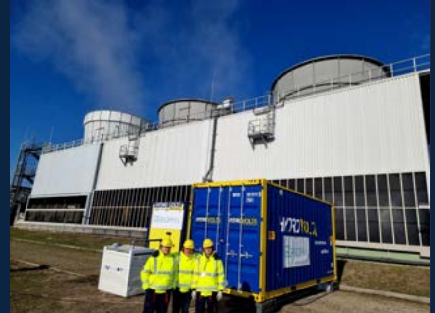
Industrial water reuse MLD (Germany)
