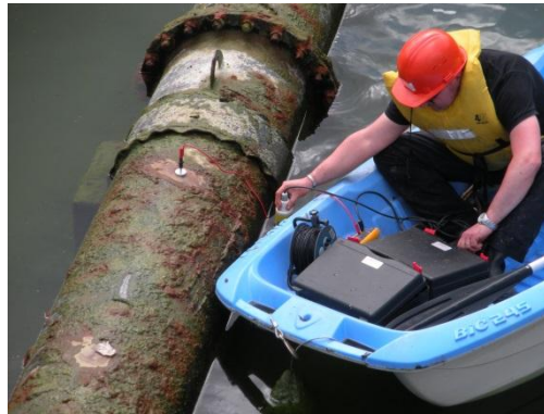
Electrochemical measurements on a pipe
