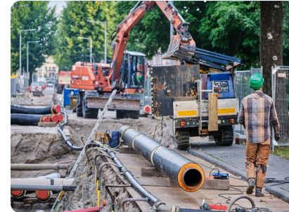
District heating connection
