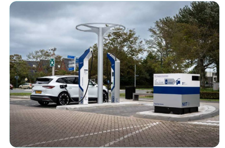
Battery buffered EV charger
