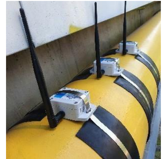
Samchully gas (2020.09) Gas pipe predictive maintenance solution
