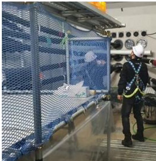
Seoul city underground collector (2020.09) Prevention of urban infrastructure-related equipment failure
