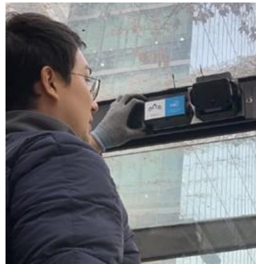
Seoul city bus station (2020.09) Environmental conditions monitoring and display
