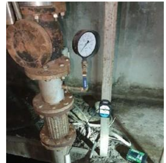
Gangwon Inje 3821 Military Unit (2020.10) Septic tank IoT management solution
