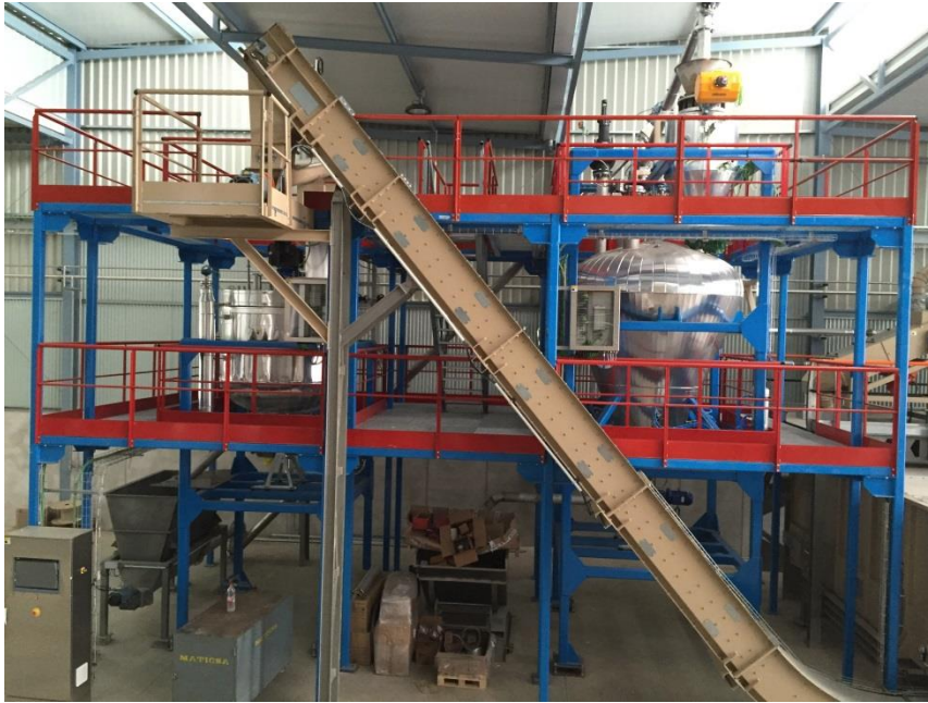
Steam Cooking and Steam Explosion reactors
