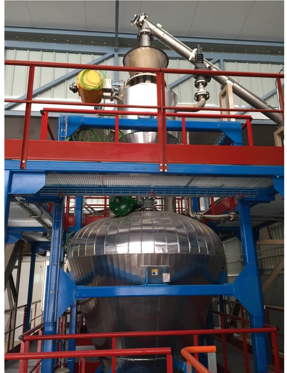
Detail of Steam-Explosion reactor and Expansion vessel
