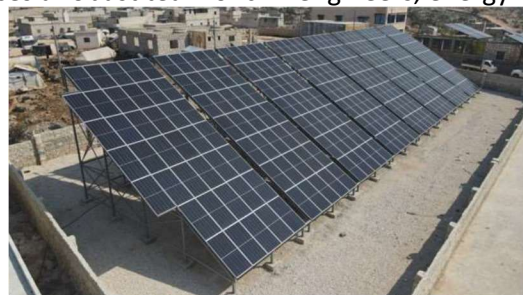
Solar power plant for water station in another CP
