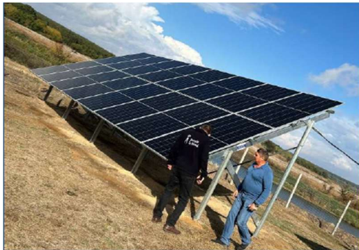
PIN Solar Power for Water System in Remote Villages. Southern Ukraine (2025)
