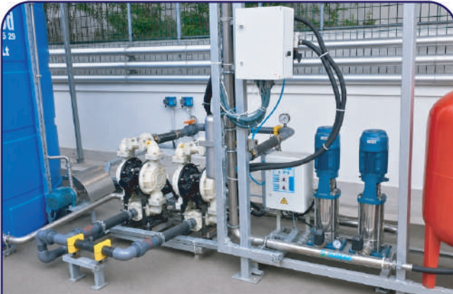
KLOR POMPA GRUBU CHLORINE DOSING PUMP SKID
