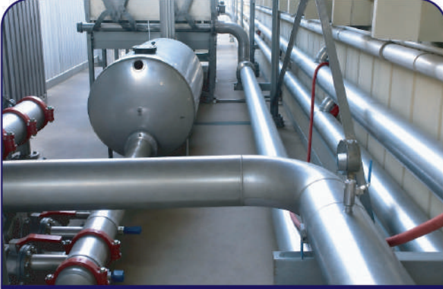
PVC ENJEKSİYON SU SOĞUTMA HATTI PVC INJECTION WATER COOLING LINE
