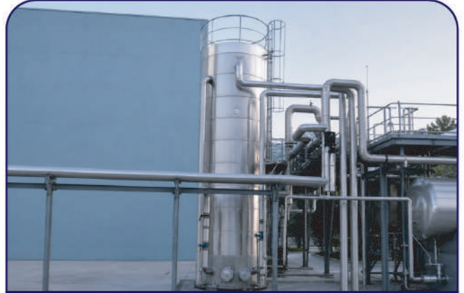
SICAK SU BALANS TANKI HOT WATER EXPANSION TANK
