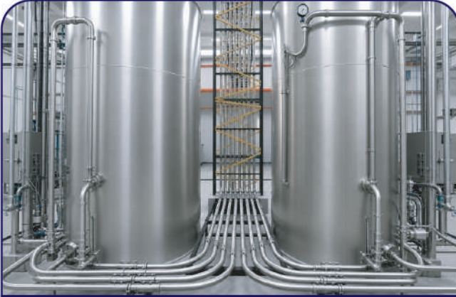
PVC GRANÜR TAŞIMA HATTI (KÖPRÜ GEÇİŞİ 2) PVC GRANULE CONVEYING LINE (BRIDGE CROSSING 2)
