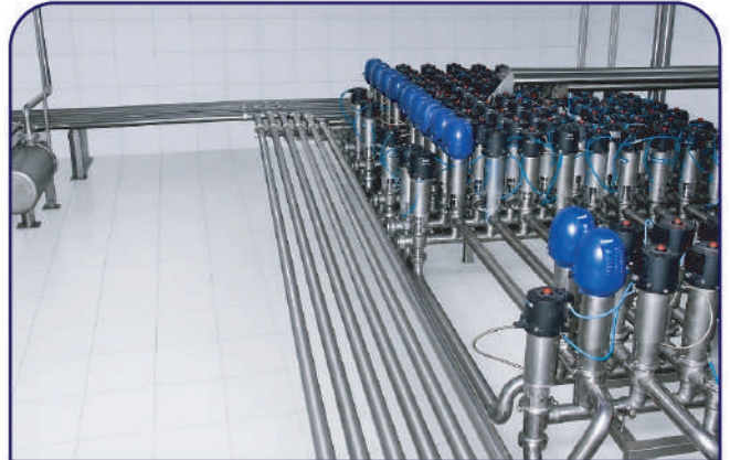
SIVI VANA TARLASI LIQUID VALVE MANIFOLD
