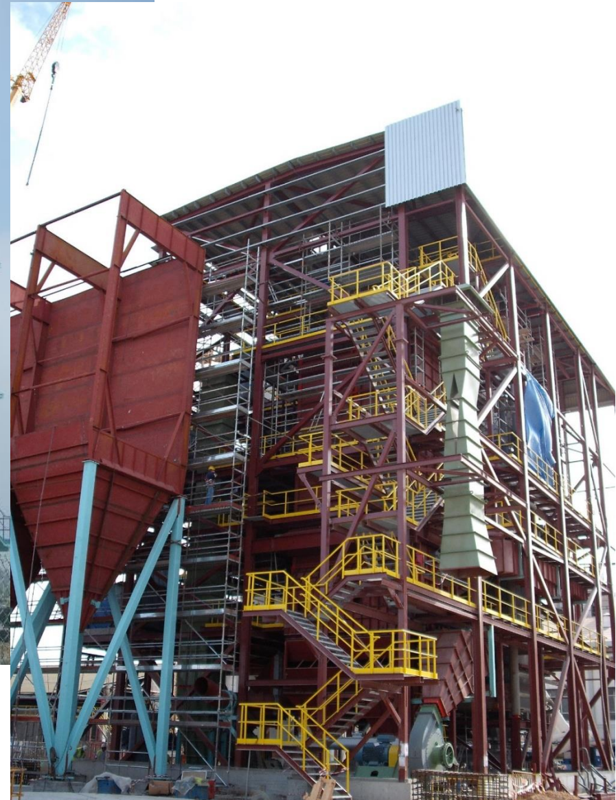
PROJECT: Biomass Power Plant PLACE: Setúbal and cacia - Portugal
