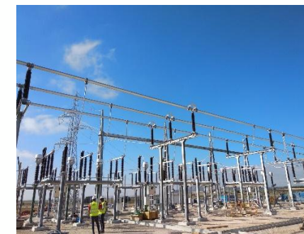
Substation and OHL Campanario 780 MVA 400 kV (Spain)
