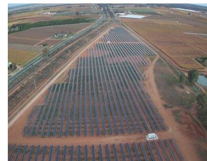
PV Francisco Pizarro 590 MW (Spain)
