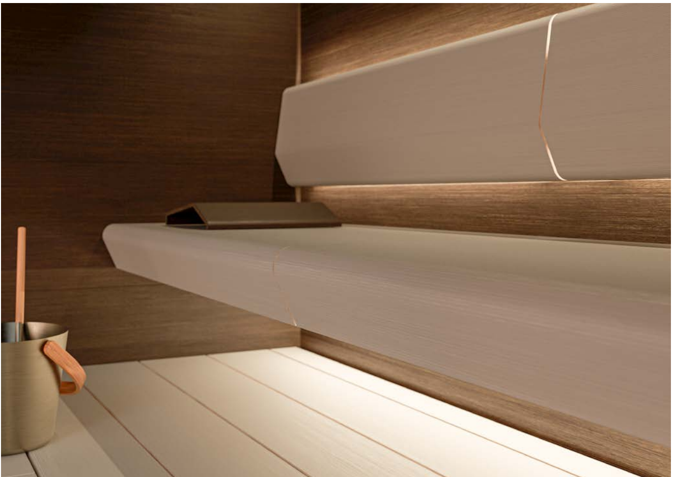
The sauna is illuminated with Sauna Linear lights both behind the backrest and under the bench.
