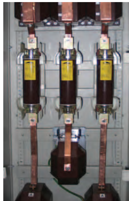
Connection in indoor switchgear, example:
