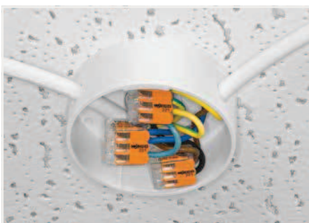
Lighting distribution in ceiling canopy
