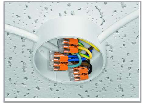
Lighting distribution in a ceiling canopy
