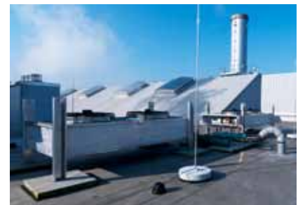
Insulated lightning protection on roof fittings
