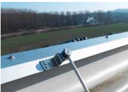
A parapet wall connected to the lightning protection system
