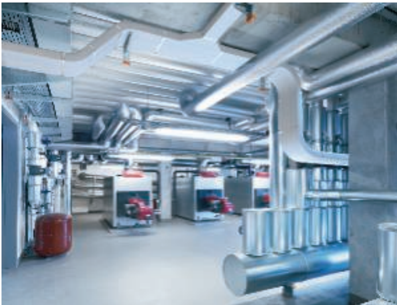
Industrial use of cable bandages
