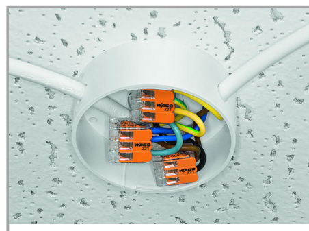
Lighting distribution in ceiling canopy
